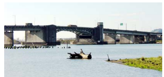
The Chehalis River Bridge provides access between South Aberdeen/Cosmopolis and US 12/downtown Aberdeen.
